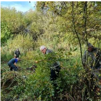
Using a winch to drag the strong roots of the willows from the middle of the canal.
