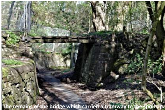
The remains of the bridge which carried a tramway to the spoil tip.
